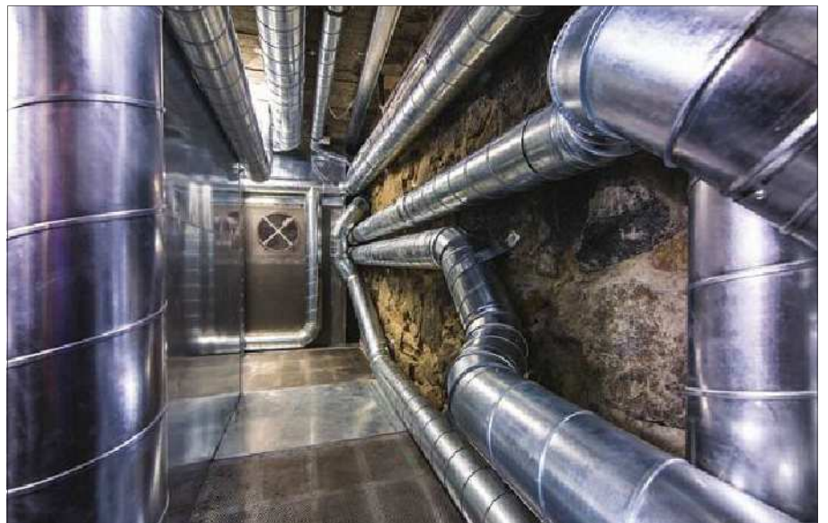
An accurate record of ventilation systems and locations of fire dampers is essential.
